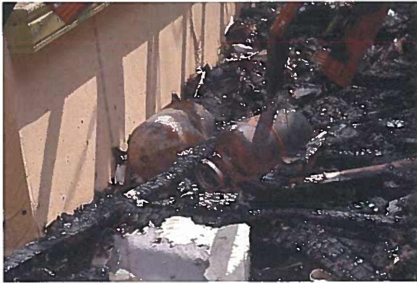
Freon Tanks Damaged by Fire
