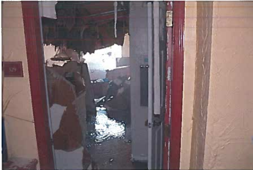
Collapse Down in Apartment 329
