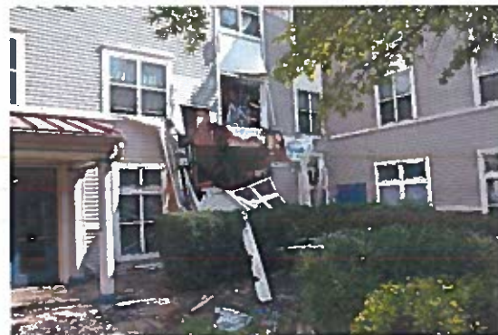
Damage from Collapse “CD” Corner
