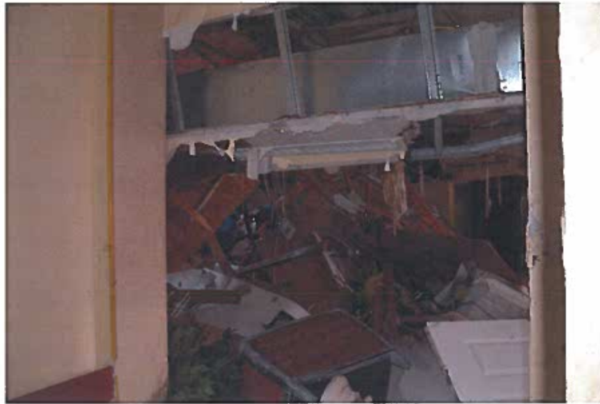
First Floor Collapse
