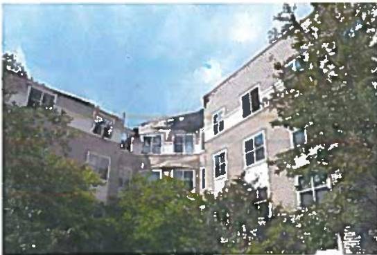
Some Burn Through “AB” Corner
