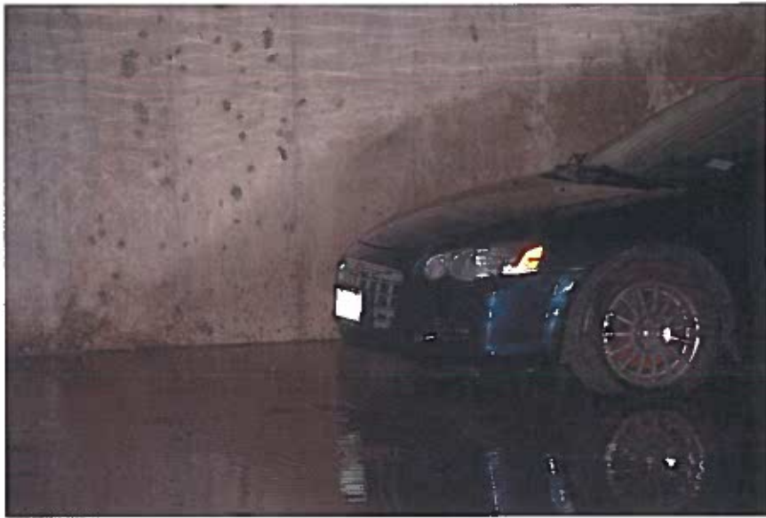
Water in the Basement
