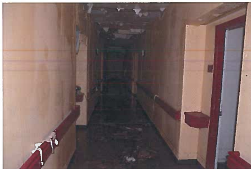
Water Damage on the First Floor
