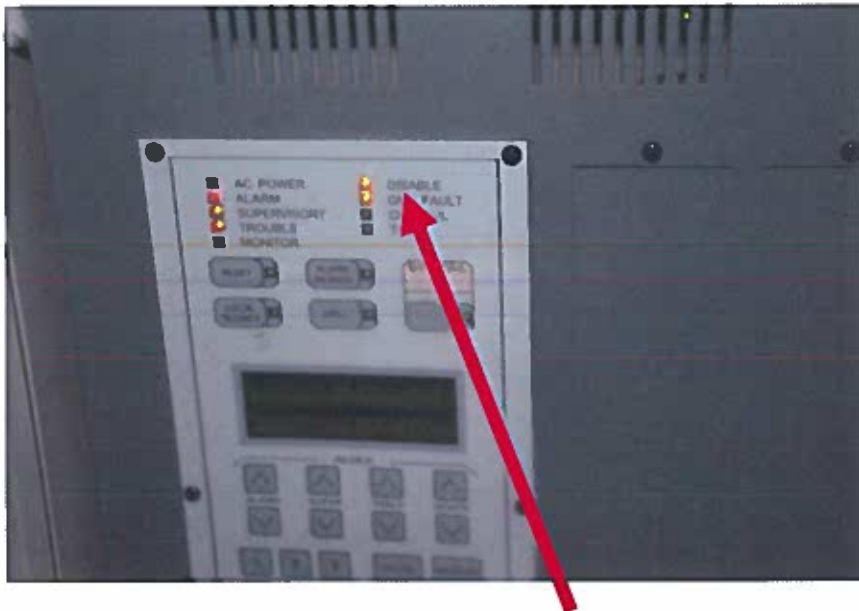
Alarm Panel with Disable Light Illuminated
