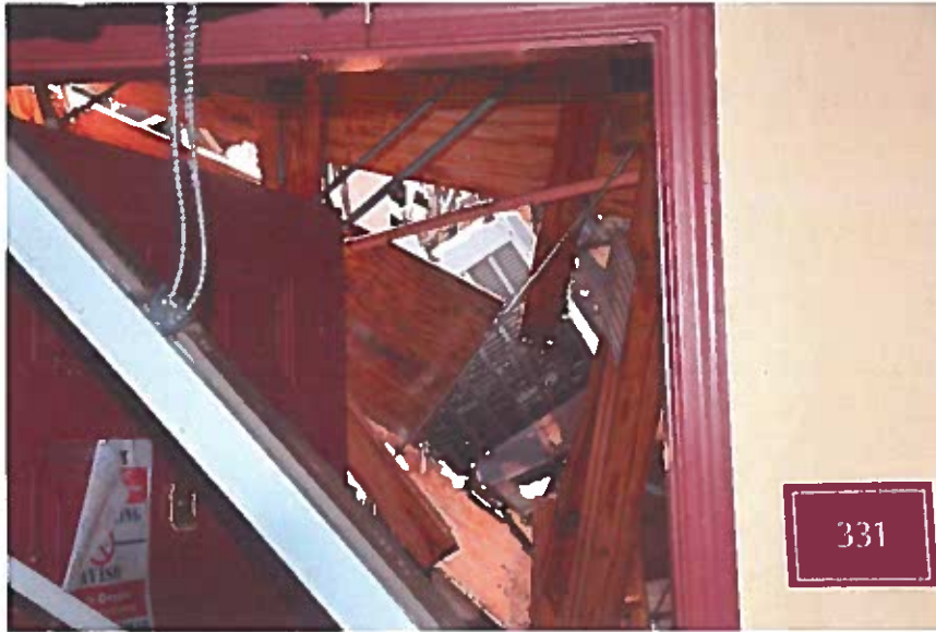
Collapse Down Through Apartment 331
