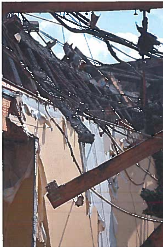
Damage above Apartment 431
