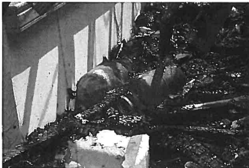
Freon Tanks Damaged by Fire
