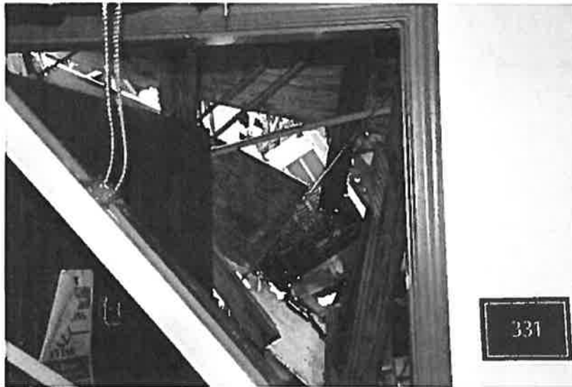
Collapse Down Through Apartment 331
