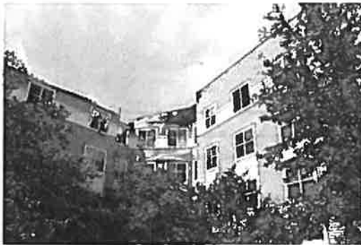
Some Burn Through “AB” Corner
