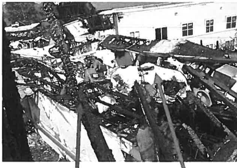
Damage to the Cockloft vs. Damage to the Flat Section
