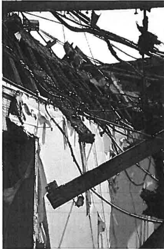
Damage above Apartment 431
