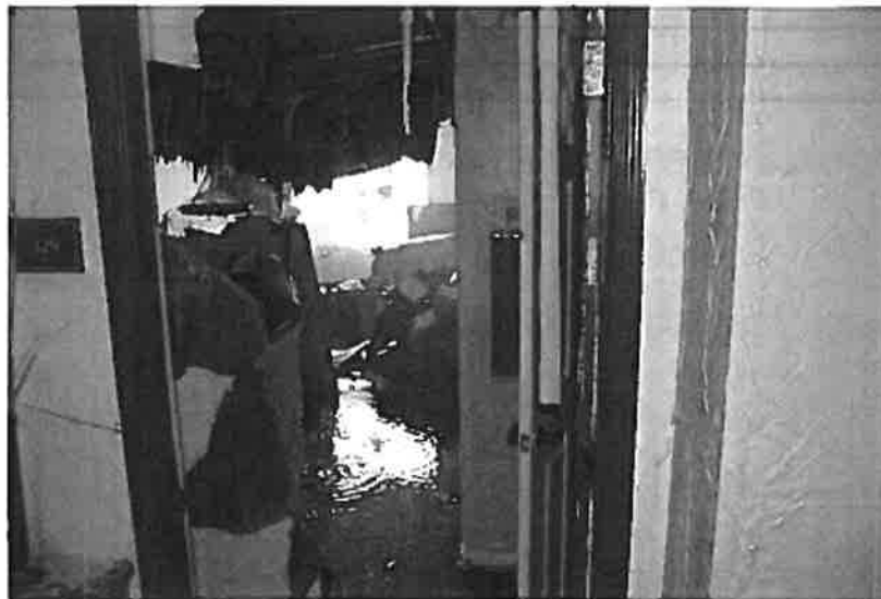
Collapse Down in Apartment 329
