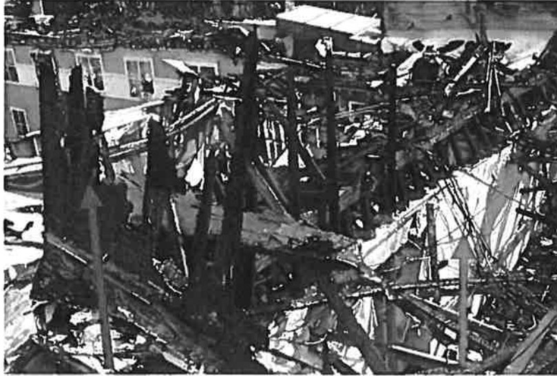
Fire Damage above the Roof Line & No Fire Damage Below
