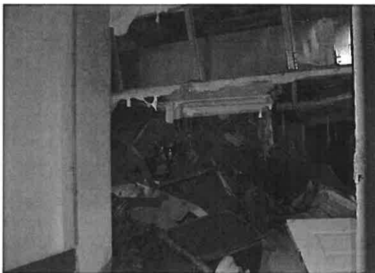
First Floor Collapse
