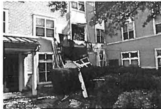
Damage from Collapse “CD” Corner
