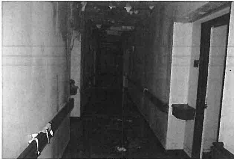
Water Damage on the First Floor
