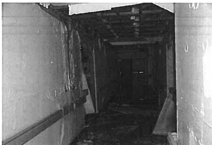
Collapse and Water Damage on the Second Floor
